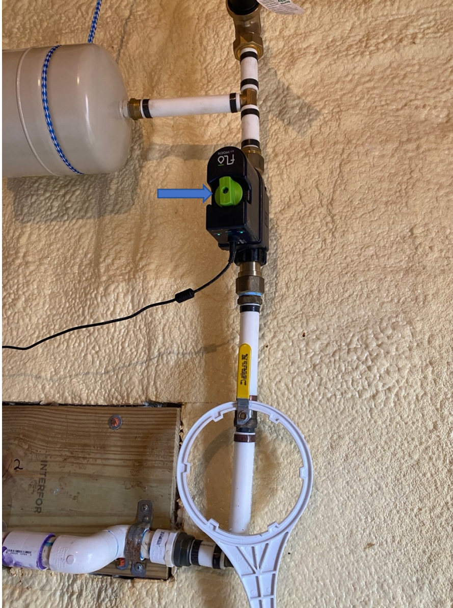
Photo #1 showing the cut off knob on the Flo by Moen unit
