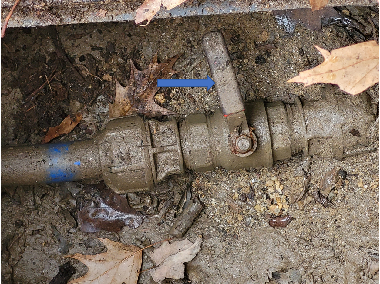
Picture 2: showing water lever in the off position on the main line into the house (located in the junction box at the house)
